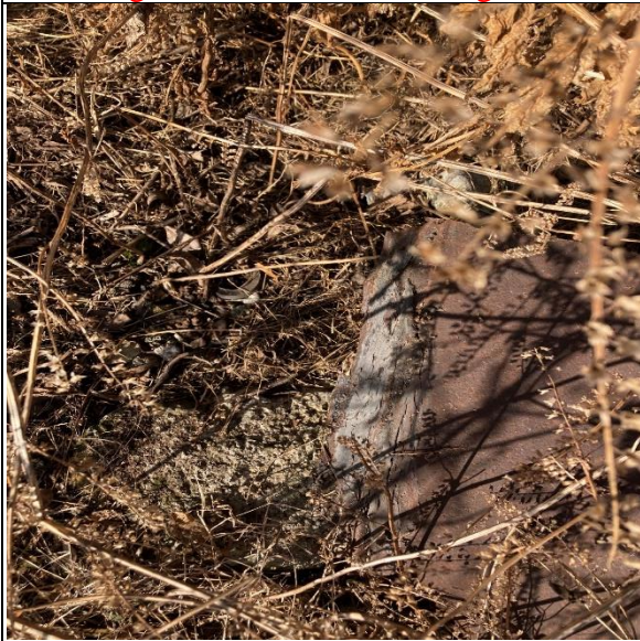
Building 1 – Asbestos containing seam tar
