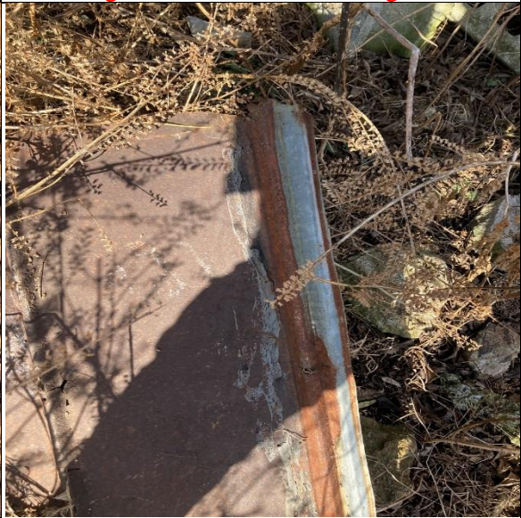
Building 1 – Asbestos containing seam tar
