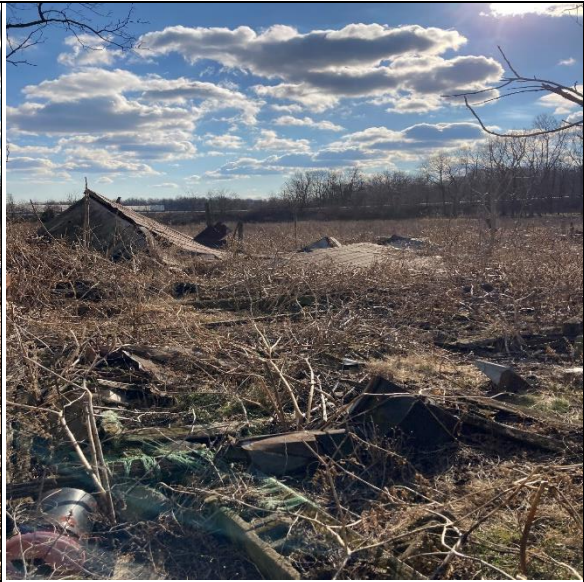
Building 1 – Asbestos containing seam tar
