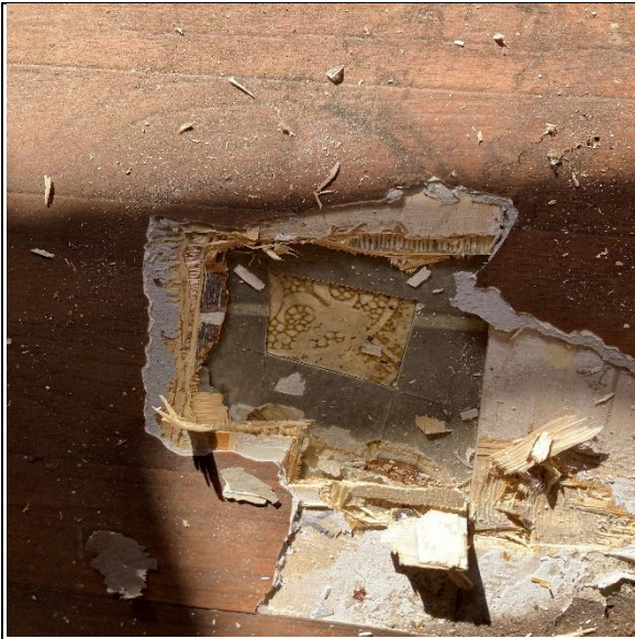
Asbestos containing yellow design sheet flooring base layer in kitchen
