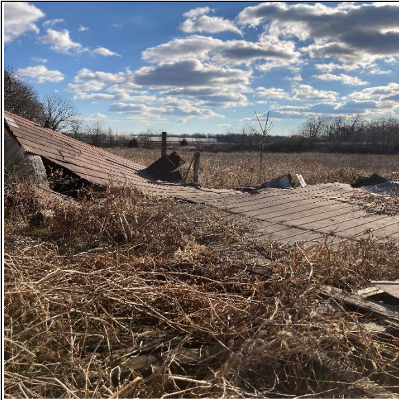
Building 1 – Asbestos containing seam tar
